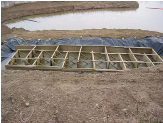
Figure 5: Mixing Chamber completed 2006
