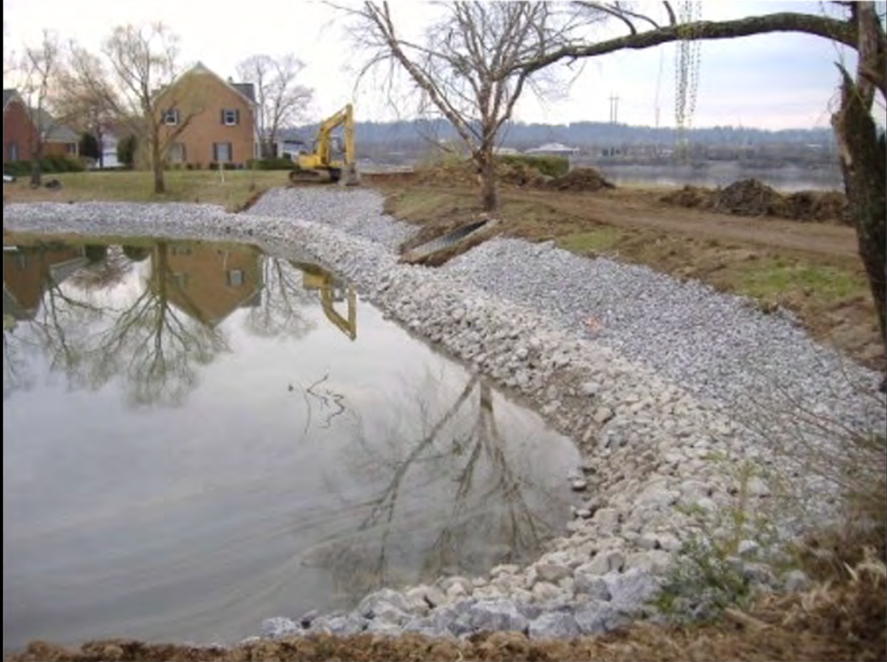
The Mudmats in the photos supported 17 Tandem axle dumps, 6000 gallons of fuel deliveries, The trackhoe and 2 skid loaders for 7 days during the winter and still held up. They were reused on another project
