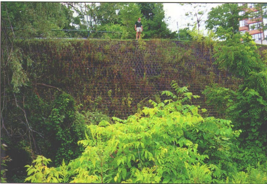
The Geoweb cellular confinement system successfully used at the Kressview Springs condominium project.
