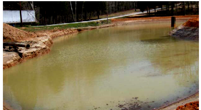
The dredge spoils discharged into the stilling pond through the pipe on the left and discharged through the riser pipe on the right.
