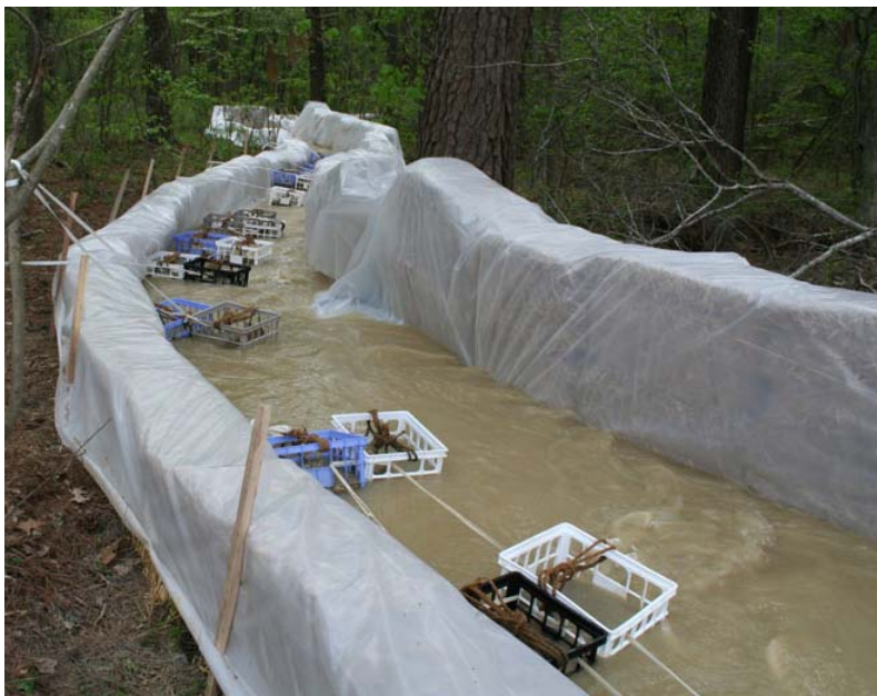
The soil-specific Floc Logs were secured into plastic crates in the mixing/reaction portion of the treatment system where the polymer would react with suspended sediment.
