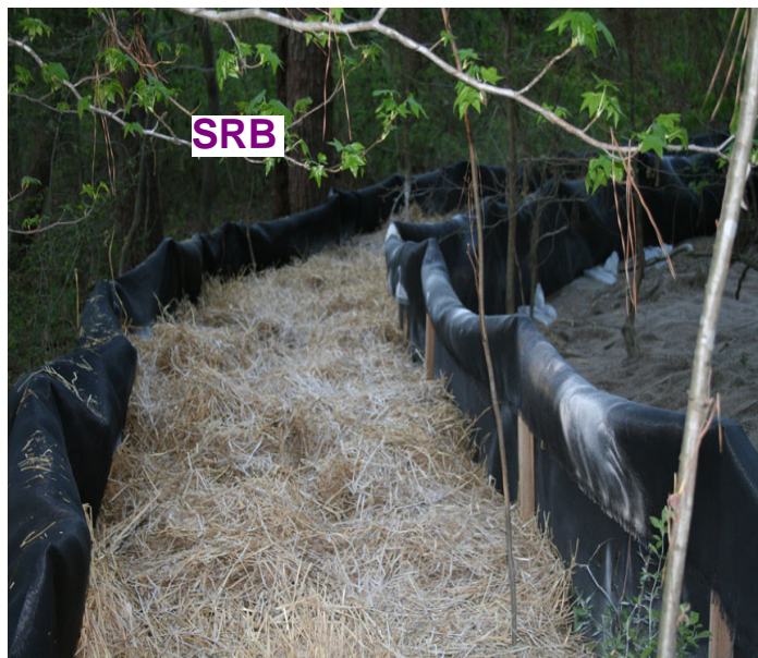
The treated water passed across the jute dispersion field before passing through the SRB (sediment retention barrier) filled with straw and polymer where final polishing occurred.
