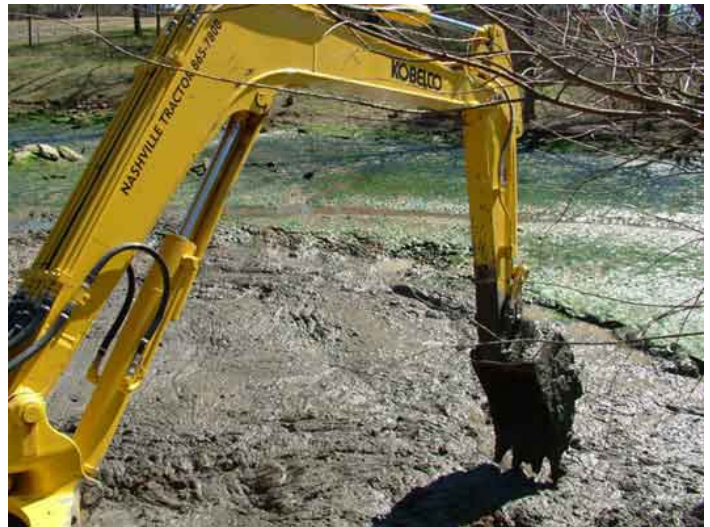
APS Silt Stop solidified the sediment for easier removal.
