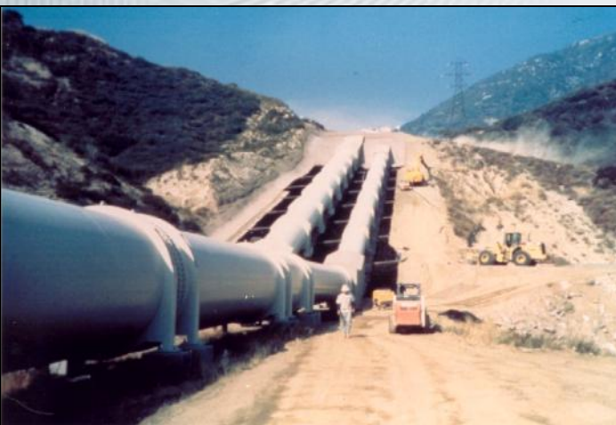
Prior to placing the concrete infill, the GEOWEB® system is installed along the base of the pipelines.
