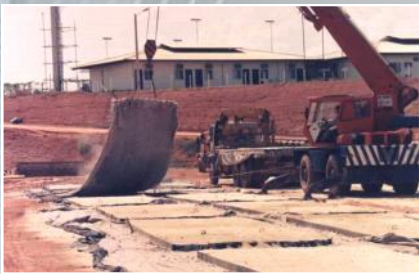
Top Photo: Lifting the flexible GEOWEB sections after the concrete is cured in preparation to transport.
