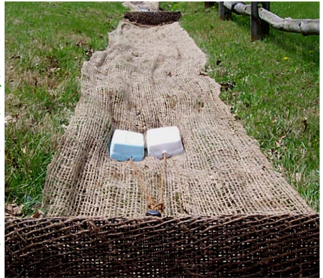
Floc Logs Treating Stormwater in an open ditch treatment train.
